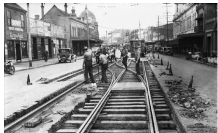
Re-laying tram track with the earlier wooden block road foundations exposed. Source: Newcastle Herald.
